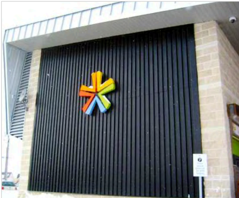
Figure 99: Solar wall on Assiniboine Credit Union, 2659 Pembina Hwy, Winnipeg 131
