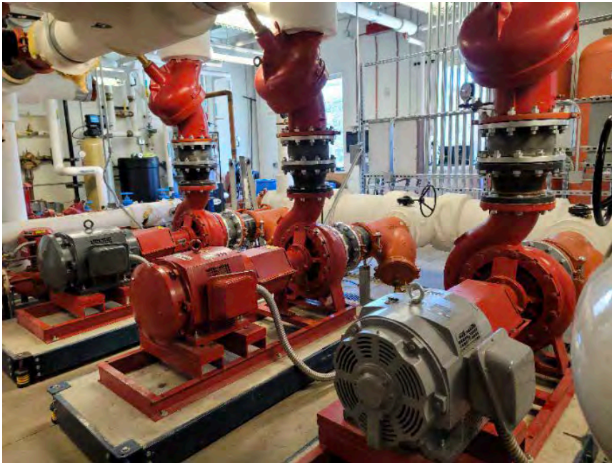
Figure 94: Central Pumping Station in Colorado Mesa University's Wubben Science Hall 121
